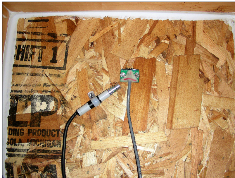
Figure 8. Instrumentation at top of cavity recording moisture content, relative humidity, and temperature.
