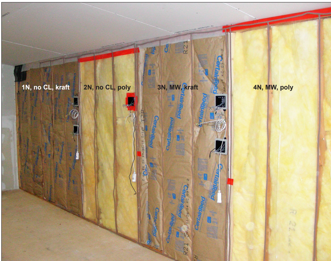
Figure 6. Northwest interior corner of test structure with wall cavities insulated before drywall installation (CI, continuous insulation; MW, mineral wool).
