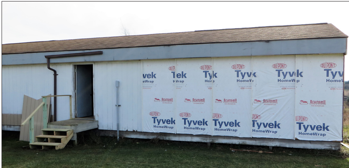
Figure 4. Northwest corner of test structure before installation of exterior insulation. The right-most section is not an instrumented section.
